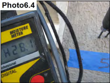
Probe 5 elevated moisture
