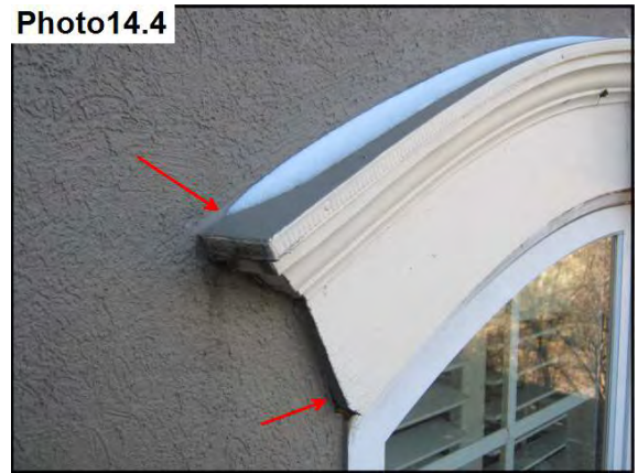
Head flashing installed but gaps at trim.
