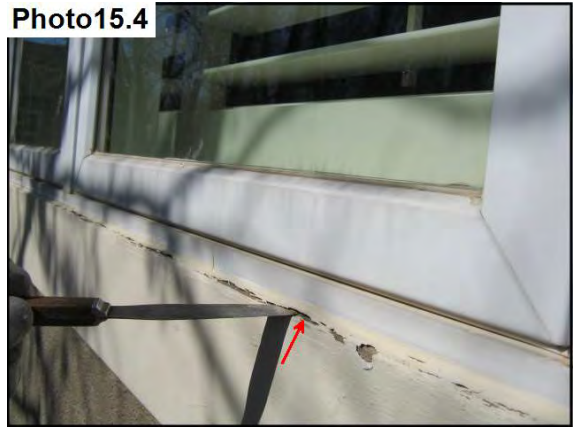
Sealants too thin to be effective.
