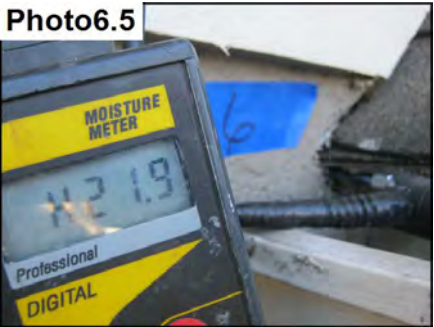
Probe 6 elevated moisture
