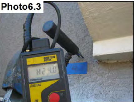
Probe 4 elevated moisture
