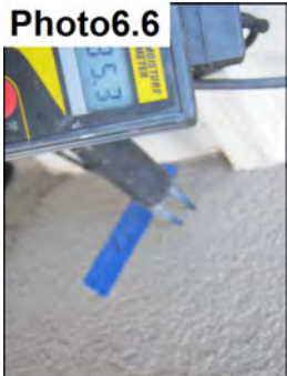
Probe 7 elevated moisture
