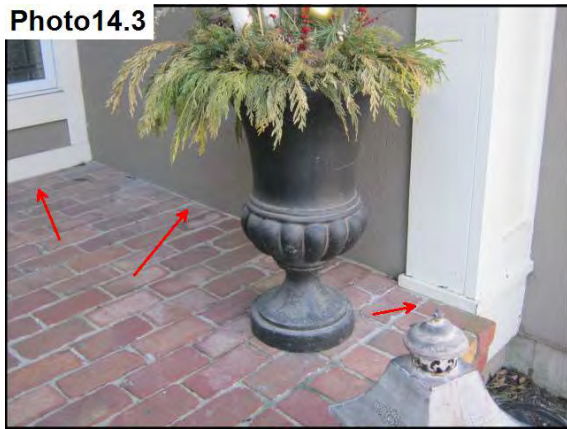
Two inch gap required.
