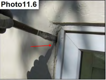
Gaps at joints
