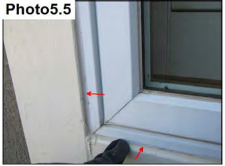
Thin sealant visible.
