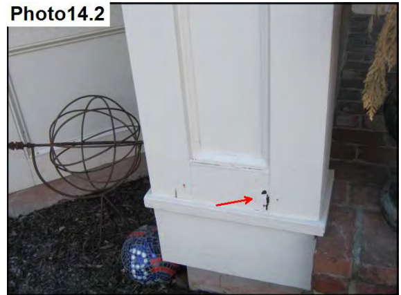
Wood rot at column
