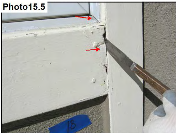
Wood rot site 18
