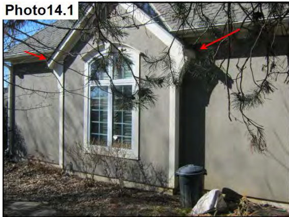
Open gap at roof wall.
