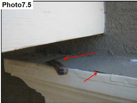
Top column flashing not sealed.
