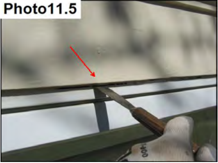
Gaps at wood trim
