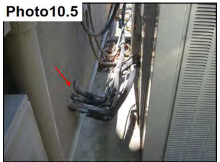
Penetrations not sealed
