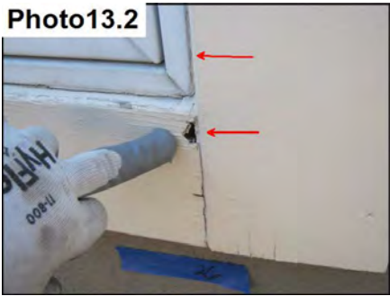
Wood rot, thin sealant.
