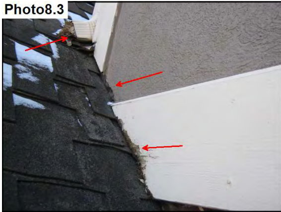
Trim/EIFS in contact with roof shingles.
