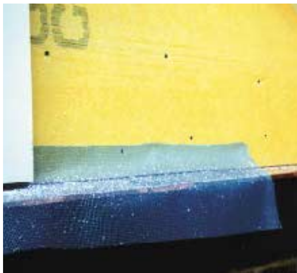
Figure 5. Headers and other horizontal surfaces must be protected with flashing. In this case, the damaged EIFS system has been stripped off, and a waterproof fiberglass-faced gypsum board screwed to the studs. The EPS board is attached to the sheathing with adhesive. Once the reinforcing mesh has been turned up at the front, the bottom edge of the sheet will receive a layer of basecoat.
