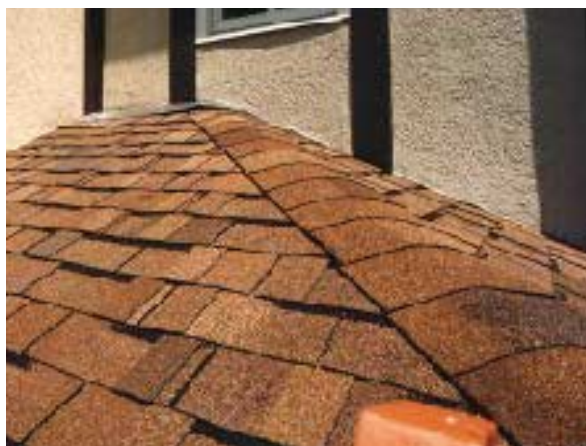
Figure 6. Contrary to the manufacturer's recommendation and common sense, the EIFS applicator butted the edge of the polystyrene directly against the roofing, with no caulk space or counterflashing.
